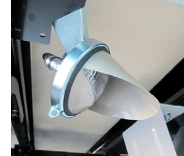
88 路肩灯 [白熱灯]
